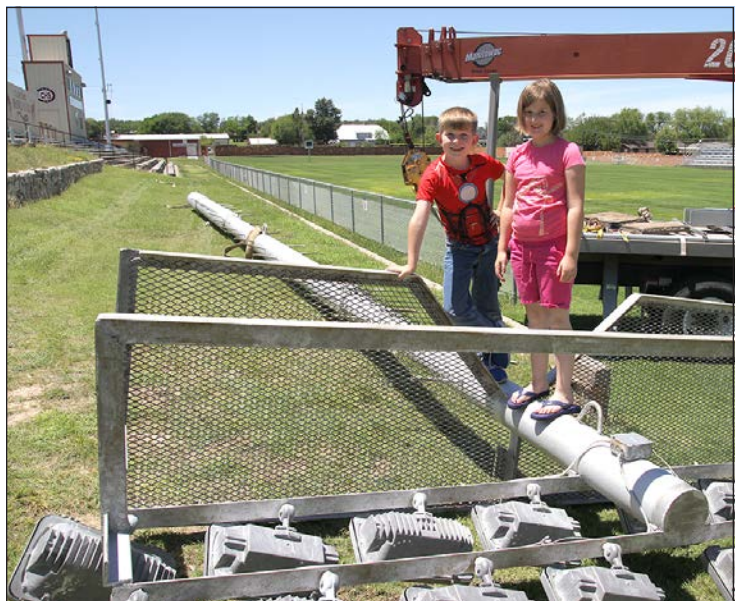
Ben and Ella Estlack stand at the top of one of the lights that was taken down at Bronco Stadium Monday afternoon.
