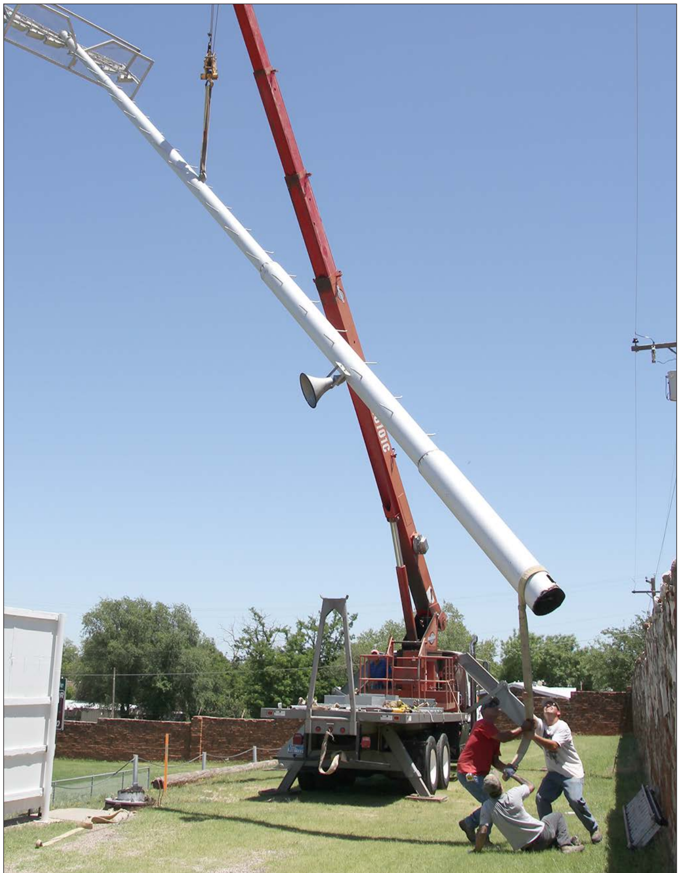
Three workers put all their weight into steadying a light pole as it comes down at Broncho Stadium Monday afternoon. The 40-year-old home-manufactured lights are being relocated to the Clarendon softball field in preparation for the installation of new modern lights at the football field. Enterprise Photo /
