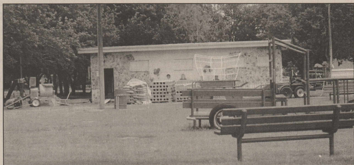
CITY CREWS ARE BUSY constructing new bathrooms at the Kennel Building in the City Park. Work is supposed to be completed in time for the July 25-26 15th Annual Seedless Watermelon Festival.
