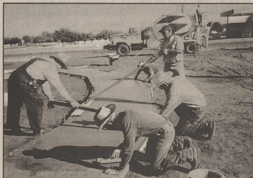
VOLUNTEER WORKERS are shown here hard at work as they finish the concrete for walkways at the new Knox County Veterans Memorial. Many Knox County residents have volunteered their time on this very worthwhile project that will honor the many men and women veterans from Knox County.
