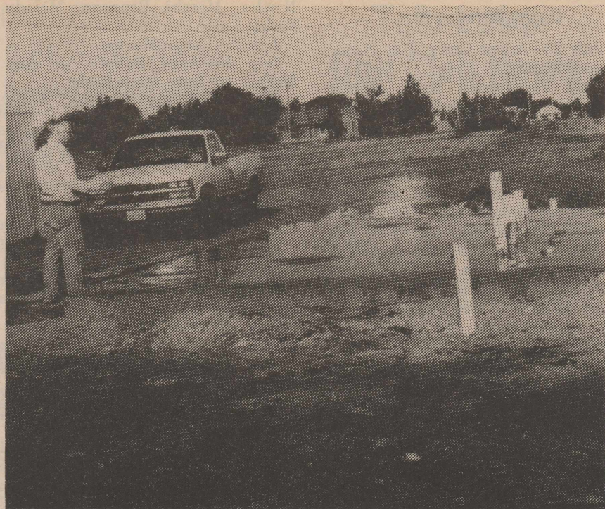
Gerald Smith was pictured where the foundation has been poured for the new concession stand and restrooms which Briscoe County Activities Association is building at the rodeo arena and ballpark. The new concession stand will open on both sides to accommodate customers at either area. The steel building is being fabricated, and will be erected by BCAA members when it arrives the first week in August. This work was begun on faith, and donations are needed to erase the indebtedness on the project. Briscoe County News Photo
