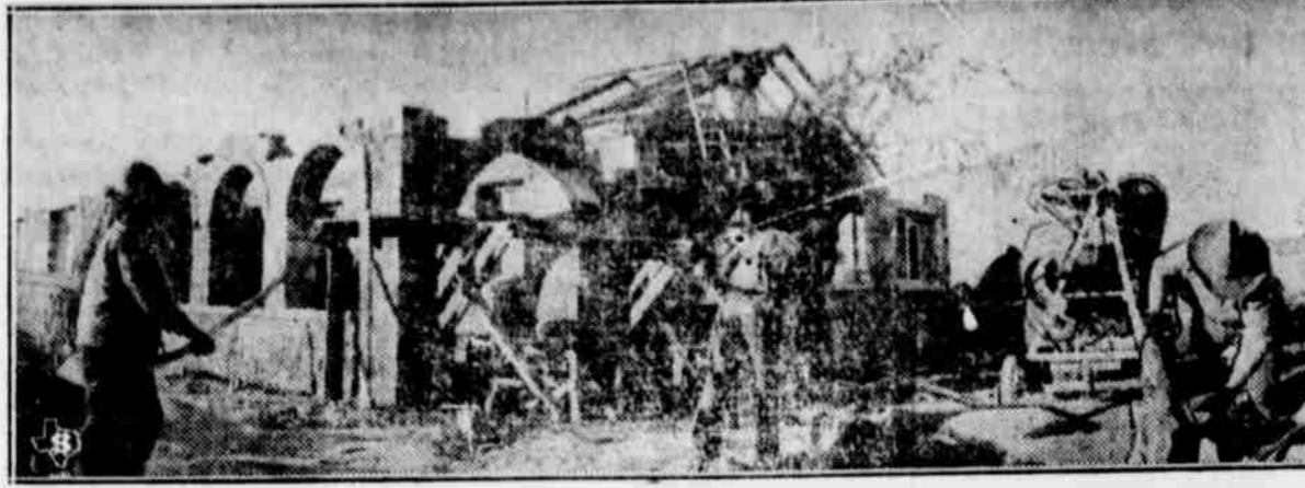
The co-operative effort of the people of Pecos county resulted in the financing of this rock county community house, pictured under construction at Fort Stockton, Texas. The house was planned with the help of the county agent and home demonstration agent, and when completed will be valued at $20,000. It will provide an excellent place for the discussion of farming problems, dinners, games and county canning operations.
