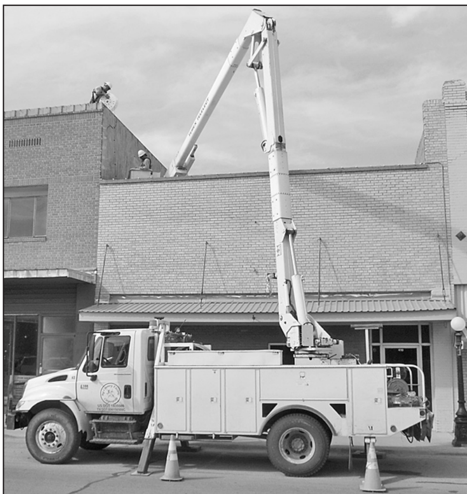
LIGHTS UP FOR HOMECOMING —Big Country Electric Cooperative crews were in Haskell on Monday re-installing the town lights that outline the buildings around the square.
