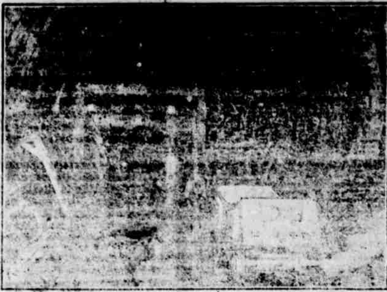
The head of one of the sections of the Ford tunnel showing the machinery used to burrow through the ground. In the foreground is one of the concrete blocks used to line the tunnel which has an inside diameter of fifteen feet.
