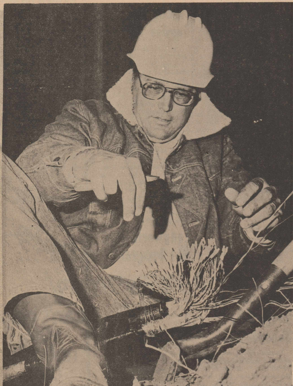
RED TO YELLOW AND GREEN TO BLUE: Southwestern Bell serviceman, Lawrence Bredemeyer connects one of the more than 400 pairs of wires severed by construction crew laying water line to new hospital. It was 11:00 P.M. when the above photograph was taken and Bredemeyer had been connecting wires since 4:30 p.m. to assure Rotan residents of un-interrupted telephone service. [staff photo]
