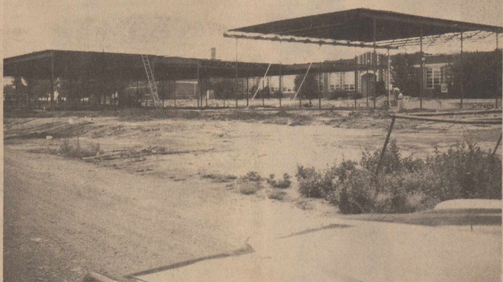
ROBY SCHOOL BUILDING: Contractors are progressing at a rapid pace in order to meet the deadline of the construction of the new Roby High School Building. This photograph was taken looking South with the Roby Elementary School behind the new construction.
