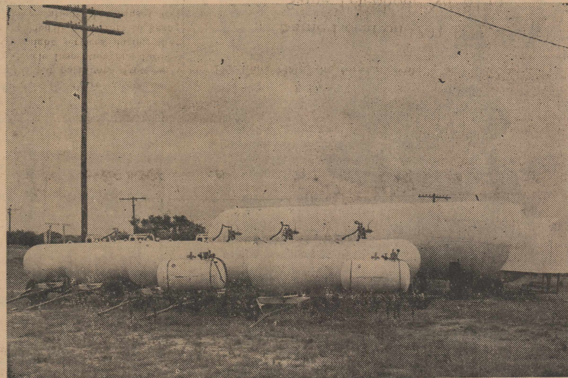
12,000 Gallon Storage System located at North Roby switch
