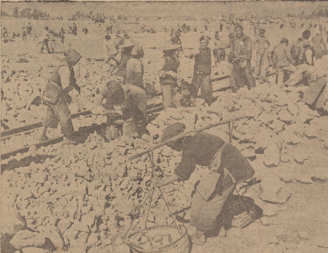
Deep in the heart of Free China, sturdy, cheerful Chinese women, boys, and oldsters are building a railroad by hand to speed the day of victory. Wearing sunbonnets and rice straw hats for protection from the hot sun, they lay track salvaged from Jap-occupied China and grade the rocky roadbed. Each stone is hewn by hand and transported by bamboo shoulder yoke.
