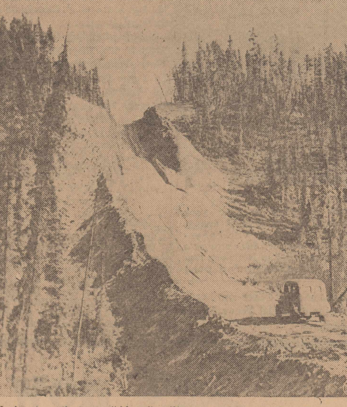
Workers on the new "Alcan" military road across Canada to connect the U. S. with Alaska are making rapid progress as they equalize topography by cutting through hilltops such as that shown above.
