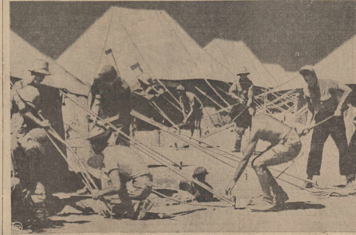
This photo may look like a shot taken as the circus arrives in town. But the scene is India and the "workmen" are U. S. troops, stripped down in the tropical heat, erecting circus-like tents that will be their homes. (Movietone News photo from NEA. Passed by censor.)
