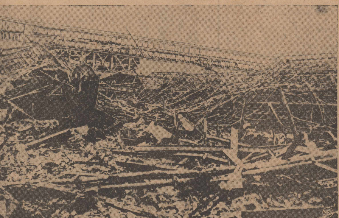
This picture is a jumble. It does not show much but it is good news for all foes of the axis for this tangled wreckage once was the great Paris Renault works. Here, until the visit by RAF bombers, vast quantities of vital German war machines were built. (Passed by censor.)
