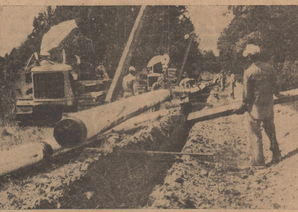
Work proceeds on pipe line from Longview to Salem, Illinois, as a step in the moving of greater quantities of oil to the Eastern coasts, from the Texas oil fields. Although it will not satisfy the full needs, the new Texas line will be of great help in that direction.
