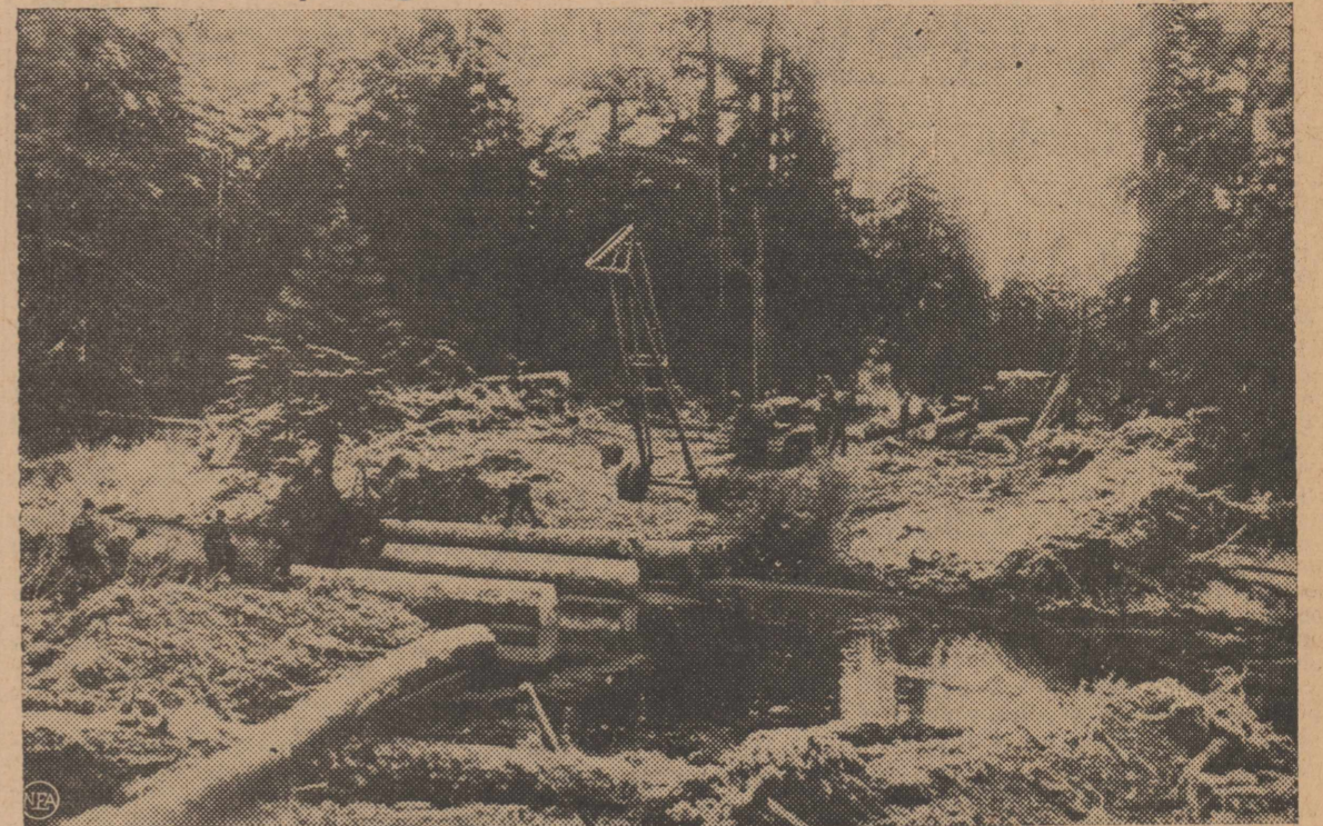
In the forests and coasts of Alaska, U. S. Army engineers are rushing roads, landing fields, barracks and docks for the defense of our northernmost outpost. These troops are using standing timber to build bridge across an Alaskan creek.
