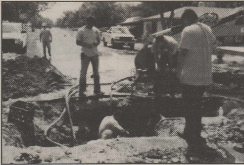
Knox City employees work inside a hole to repair a water line lead on Monday morning. The leak took place at the intersection of Fourth Street and Highway 6.
