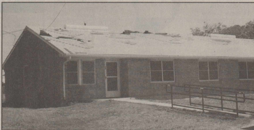
The Knox City Housing Authority was among many places in the community that suffered roof damage due to the high winds that swept through Knox County on Monday.
