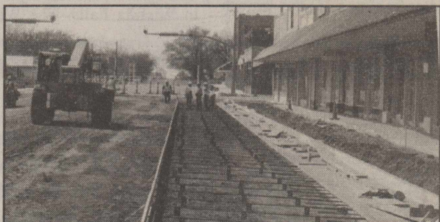
Road crews began placing the metal grid work on the northern half of Central Avenue earlier this week in preparation for pouring the new roadway.
