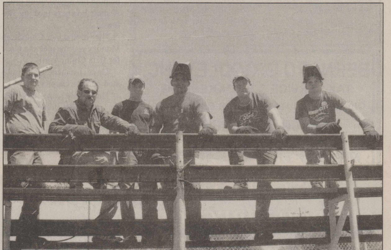
The Knox City High School Ag Mechanics classes have been working diligently on renovating the stands at the Little League Field. They have removed all of the wooden seats and replaced them with metal. Mr. Moeller commented on how well the students have worked throughout the process and is extremely proud of each and every student. Pictured l-r—Cody Trimble, Mr. Moeller, Travis Hawkins, Amos Lerma, Brandon Grimsley and Cody Wainscott. Not pictured is Joe Albus.
