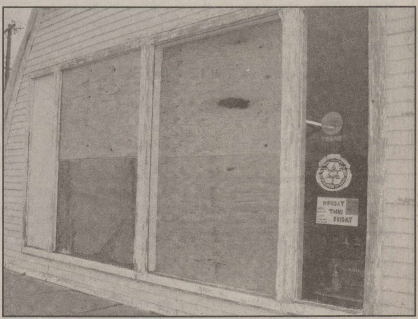
Front plate glass windows that were blown in at Jerry's Plumbing during last Friday's storm
