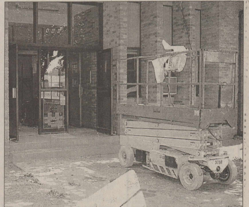
THE FRONT ENTRANCE to Knox City High School is one of the many areas receiving a facelift during the current summer renovation project underway at the high school campus. Central heat and air will replace old window units (NEWS digital photo)
