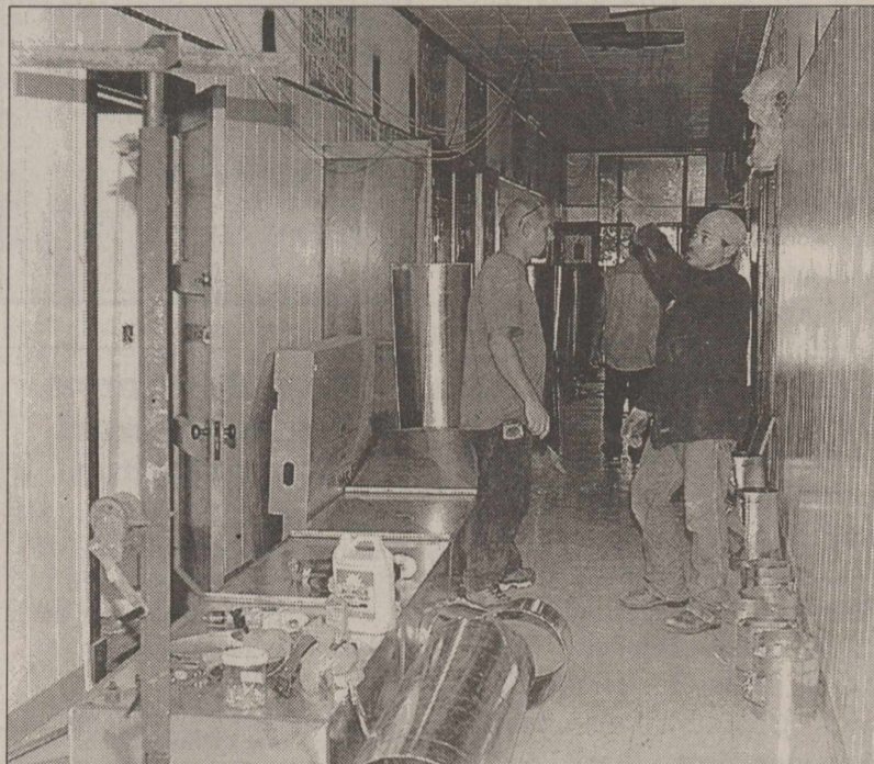
CONSTRUCTION WORKERS are hard at work in the Elementary School building as they lay out all the duct work for the new central heat and air conditioning system that is being installed in the ceiling. (NEWS digital photo)
