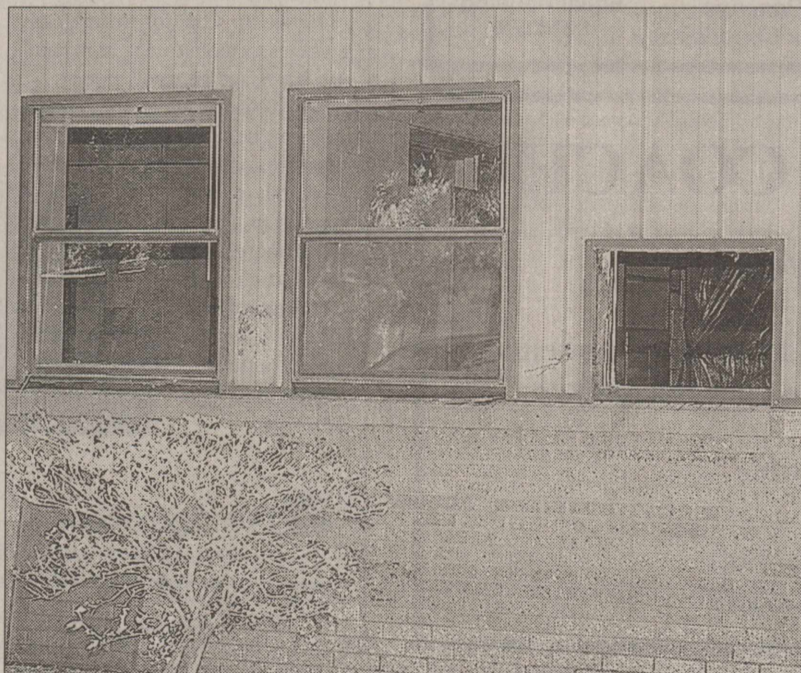
EMPTY HOLES in the walls are all that is left as a reminder of the old window units that were installed back in 1974 when refrigerated air was first introduced at the KC school campus. (NEWS digital photo)
