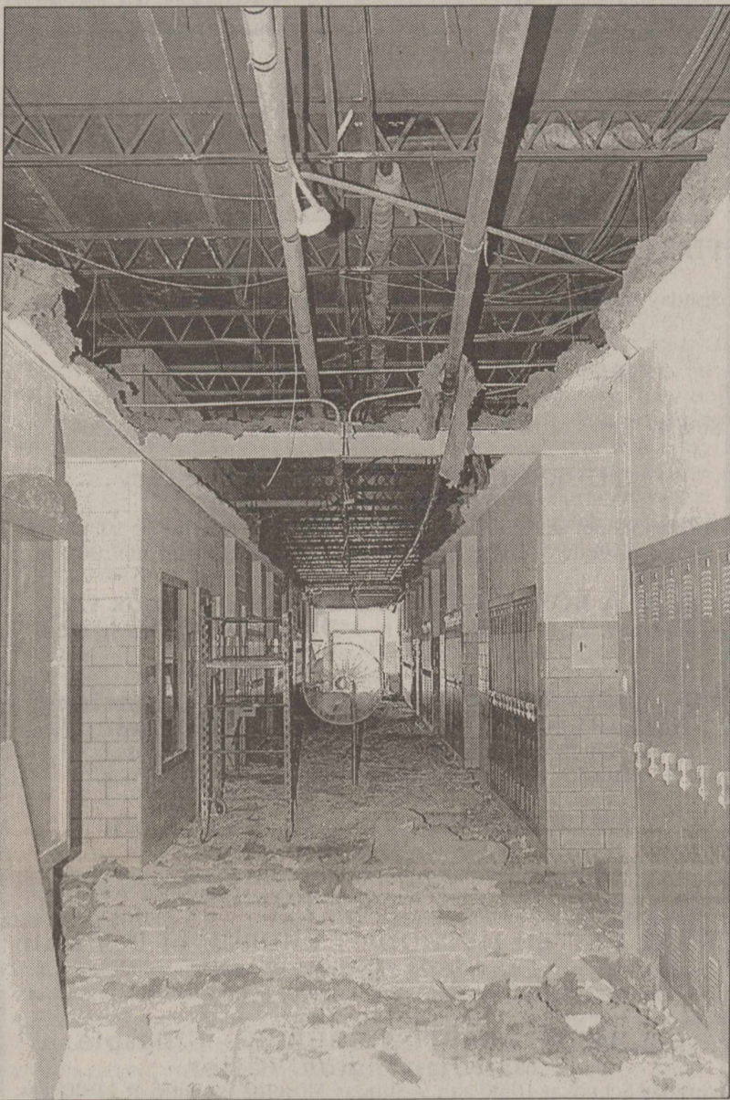
EVIDENCE OF RENOVATION is everywhere at the Knox City high School building as workers have already torn out the old cement ceiling in order to prepare the area for installation of the new central heat and air conditioning. (NEWS digital photo)
