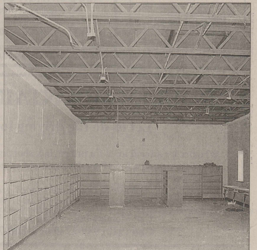
THE ONCE FULL BOOKSHELVES inside the Knox City High School Library sit empty while the ceiling inside the room has been removed as a part of the ongoing renovation project at the school. (NEWS digital photo)
