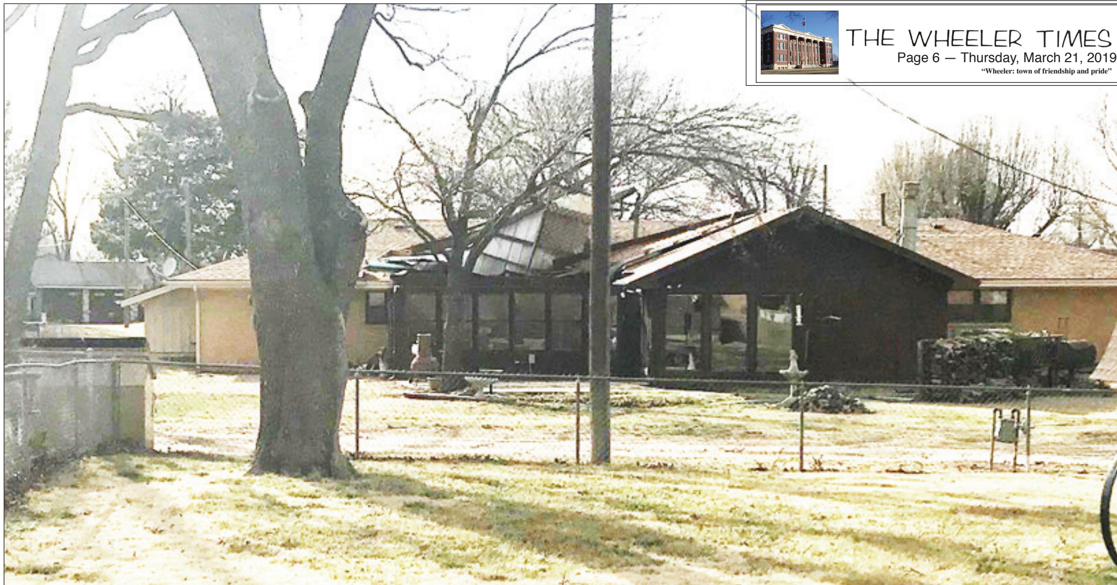
STRAIGHT WINDS TUESDAY/WEDNESDAY: Straight wind can do strange things. This is the south portion of the roof of Sharon Wright's sun room on the east side of her house on Canadian Street. During the night Tuesday, March 12-13, the roof was lifted and then folded back over the east slope of her house later when the wind shifted.
