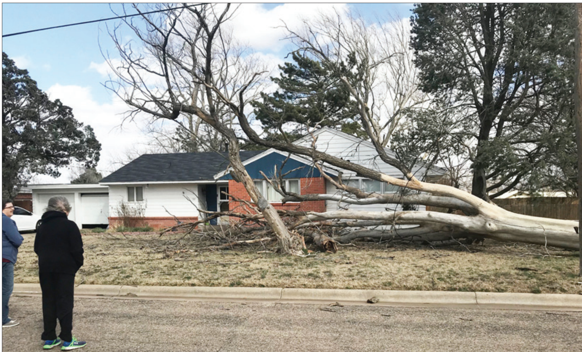
MORE WIND DAMAGE: Nancy Morrison is looking at the damage done to her home at 1111 S. Main. A neighboring tree fell, punching a hole in a gable end of her house and breaking a window. Wind gusts of around 70 miles per hour caused havoc throughout the Panhandle.
