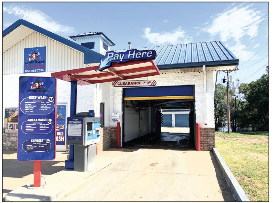
The Grime Scene Car Wash is now open for business. The former Soapy Springs property was repaired and a new drive-thru car wash system was installed.
