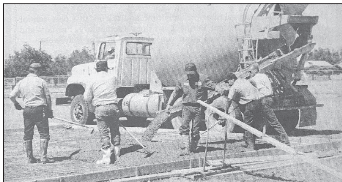
POURING HELIPAD . . . Members of the Friena Emergency Service are shown pouring the cement for the new helicopter landing pad adjacent to Parmer County Community Hospital. The cement for the new facility was donated by Panhandle Concrete. (Friena Star, Saturday, June 12, 1993)
