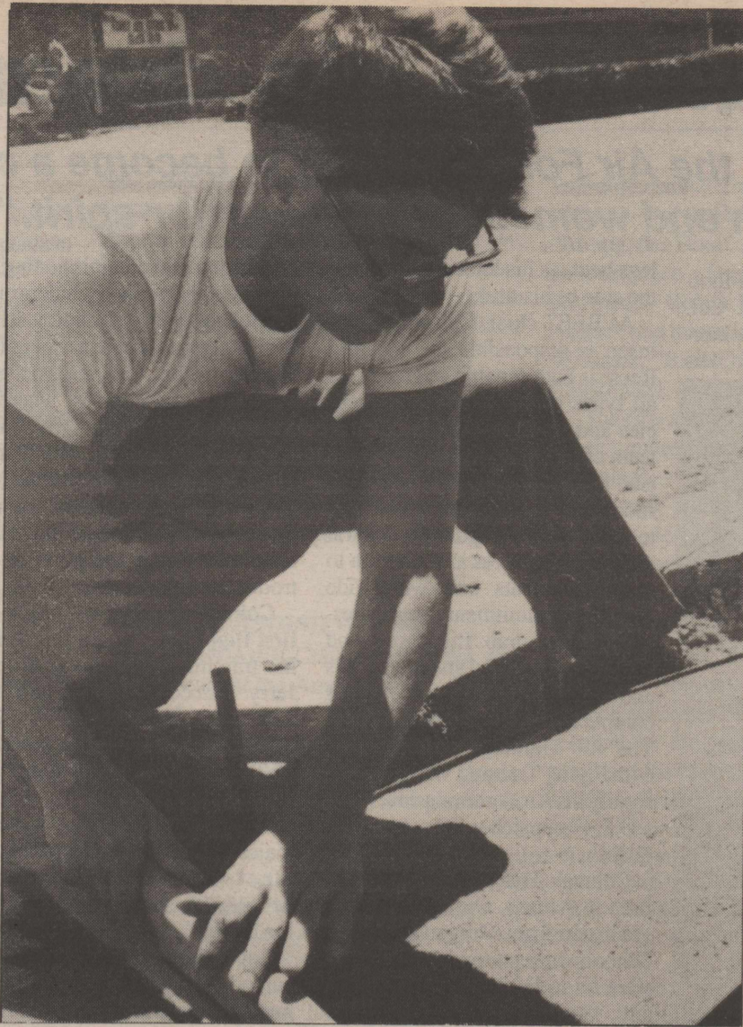
Smoothing out the lumps, A1C Stuart Jackson levels the main gate's new sidewalk. (U.S. Air Force photo by Sgt. Kimberly Nelson)
