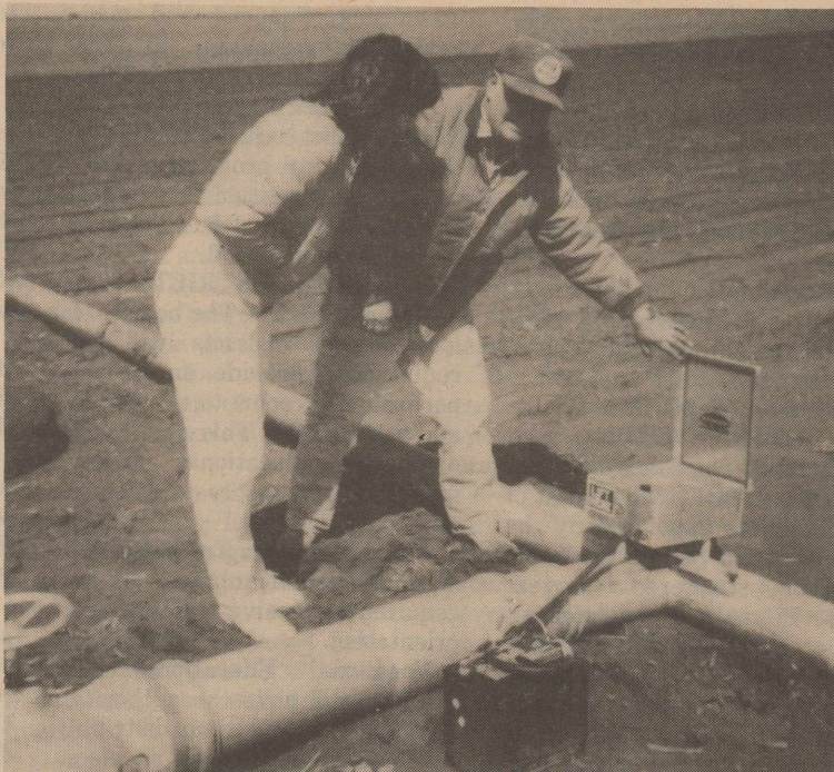
Elton Cantwell shows surge valve set-up to SCS trainee Melony Chandler.
