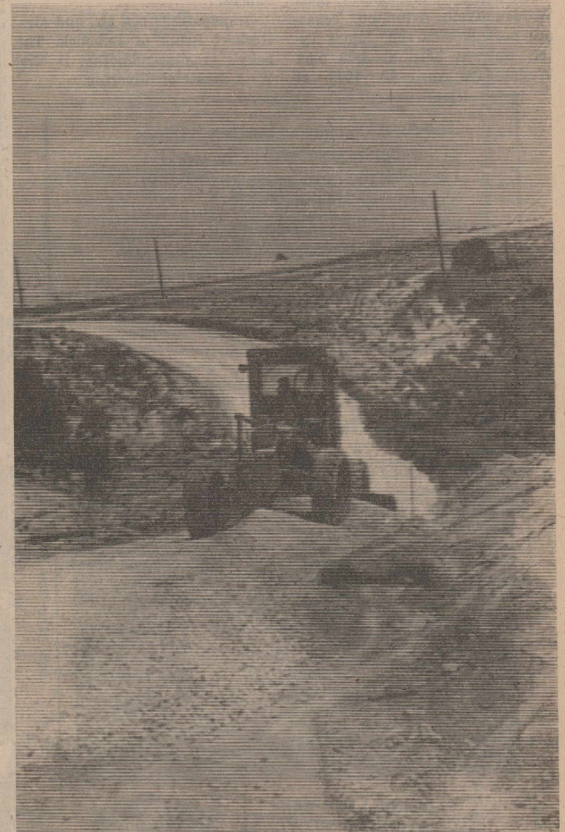
Rock is being spread on some of the roads at Lake Mackenzie, from the gate to the office and
