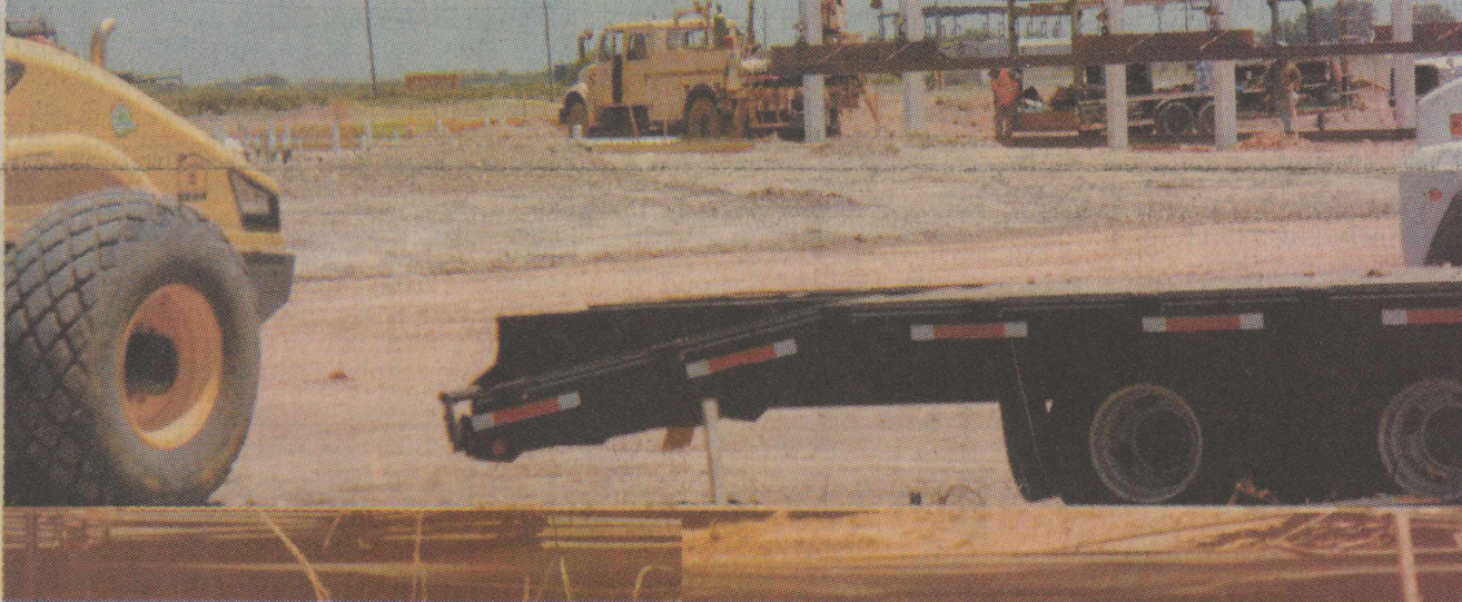
CELINDA HAWKINS | ENTERPRISE PHOTO Construction is underway at the site of The Crossing, a travel stop located at the corner of Highway 83 and 153 in Winters.
