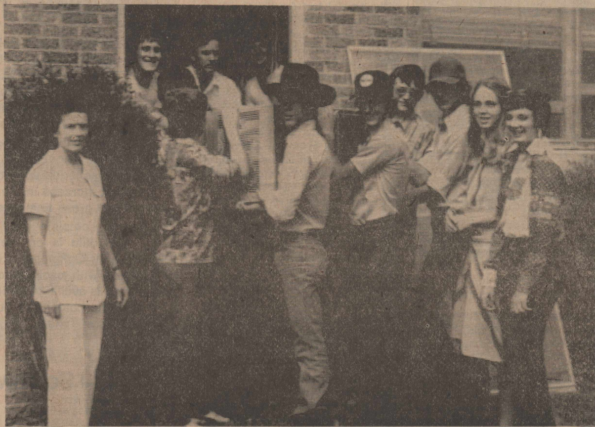
AIR CONDITIONING INSTALLED —Pictured as the school library received air conditioning units recently were Mrs. O. C. Rampley, *
