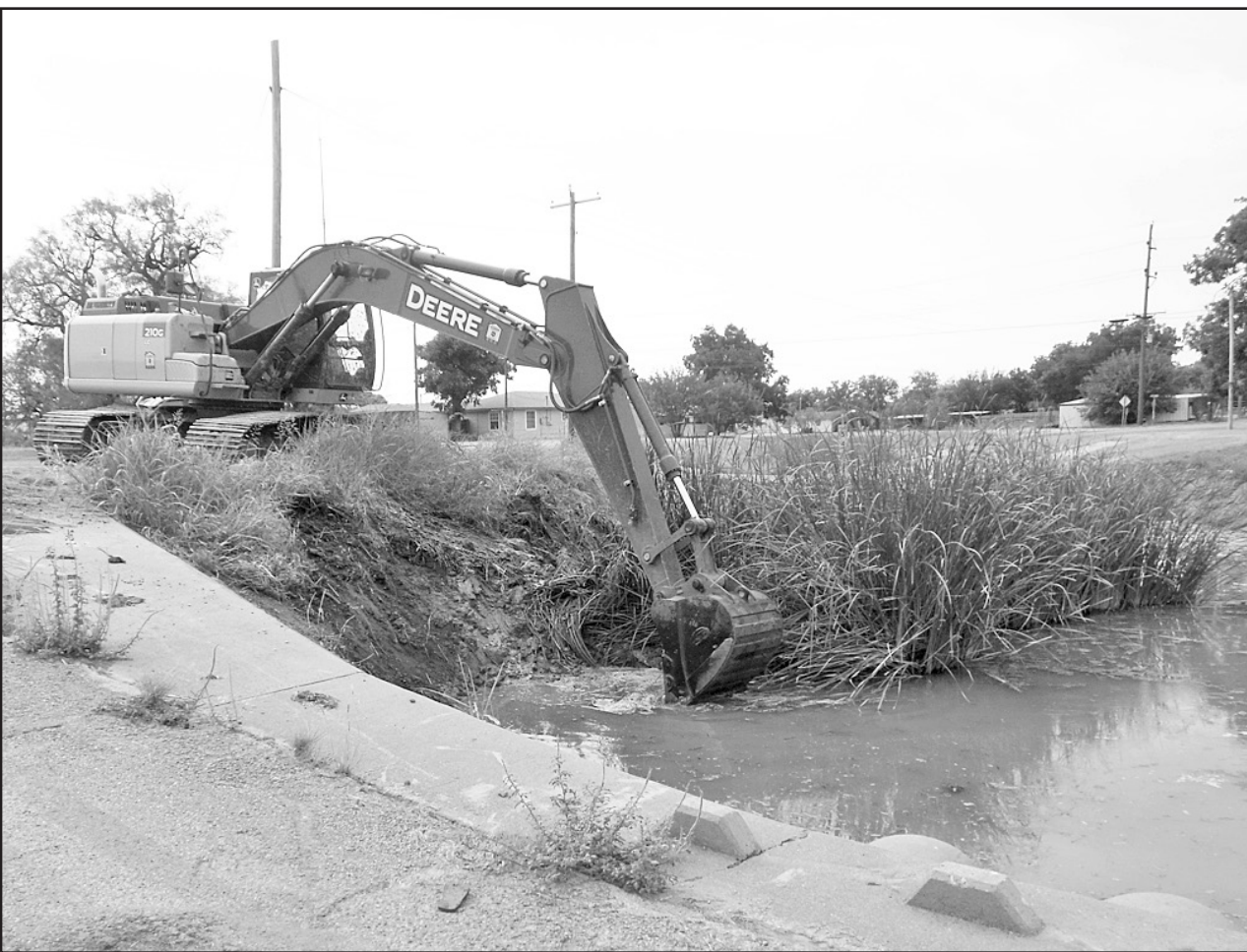
CREEK CLEANUP -The City of Haskell employees are cleaning up the creek that runs through town as time permits. The county is helping by supplying equipment for use by the work detail.
