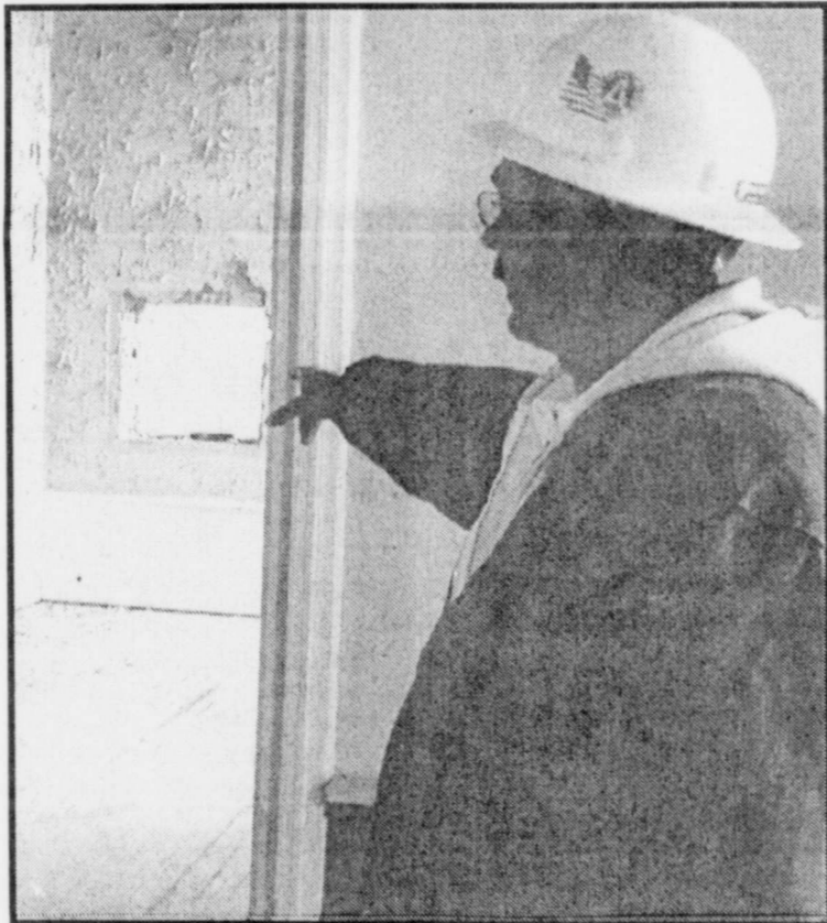
STEVE DUNN of Harrison-Walker & Harper points out the cracked paint on the walls of the Red River County Court House, which is currently under renovation. (Staff Photo by Thomas Nichols)
