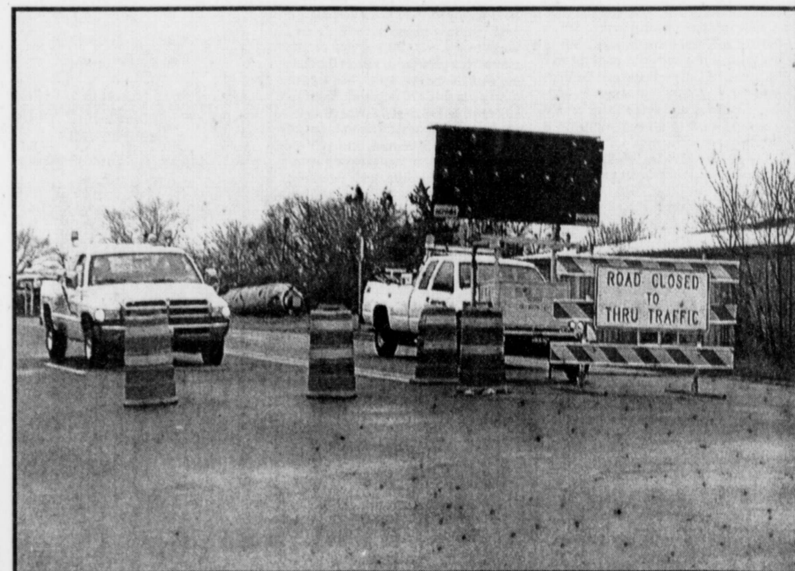
ROAD BLOCKS -were set up on Monday and Tuesday of this week on Hwy. 271 in Talco and Bogata to halt traffic going north of Talco and south of Bogata. Sulphur River overflowed it's banks sometime Sunday night and at print time was expected to drop off the highway by Wednesday morning. Hwy 37 between Hagansport and Bogata was also closed due to Sulphur's escape from its banks. On Tuesday Hwy. 37 was opened to traffic. (Staff Photo Nancy Brown)
