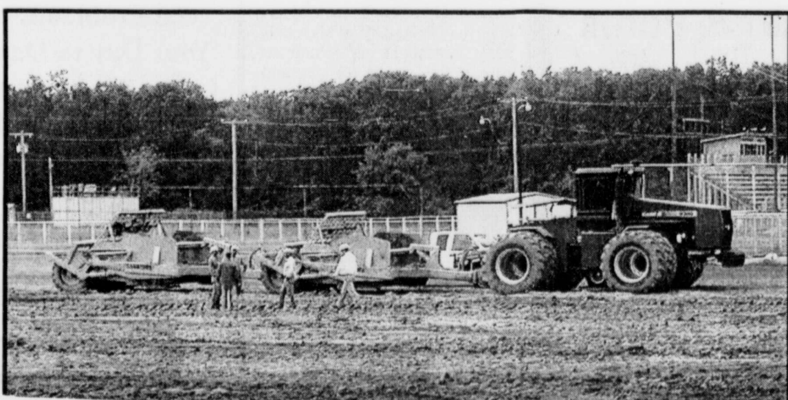
DIRT WORK-has begun on the new Rivercrest High School. The equipment was moved in last week and hopes are high to have students in the new building next year. (Staff Photo Nancy Brown)
