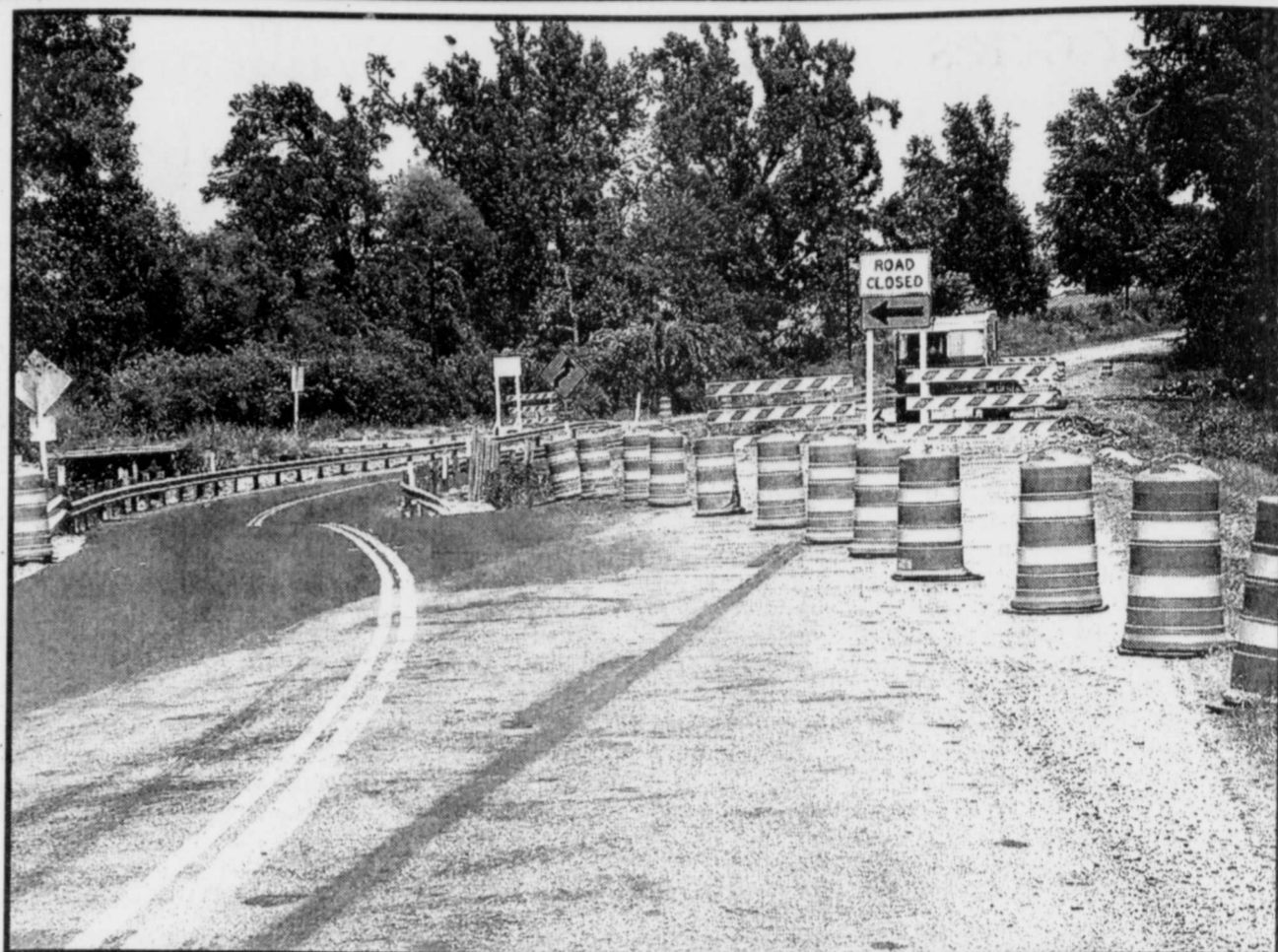
UNDER CONSTRUCTION -The old narrow bridge located just out of Bogata toward Rosalie on FM909 is being replaced. Travelers in the area are happy to see the improvement since the spot has been the scene of several accidents over the years. All drivers are advised to slow down, take care and be patient, the new bridge will soon be open. (Staff Photo Nancy Brown)
