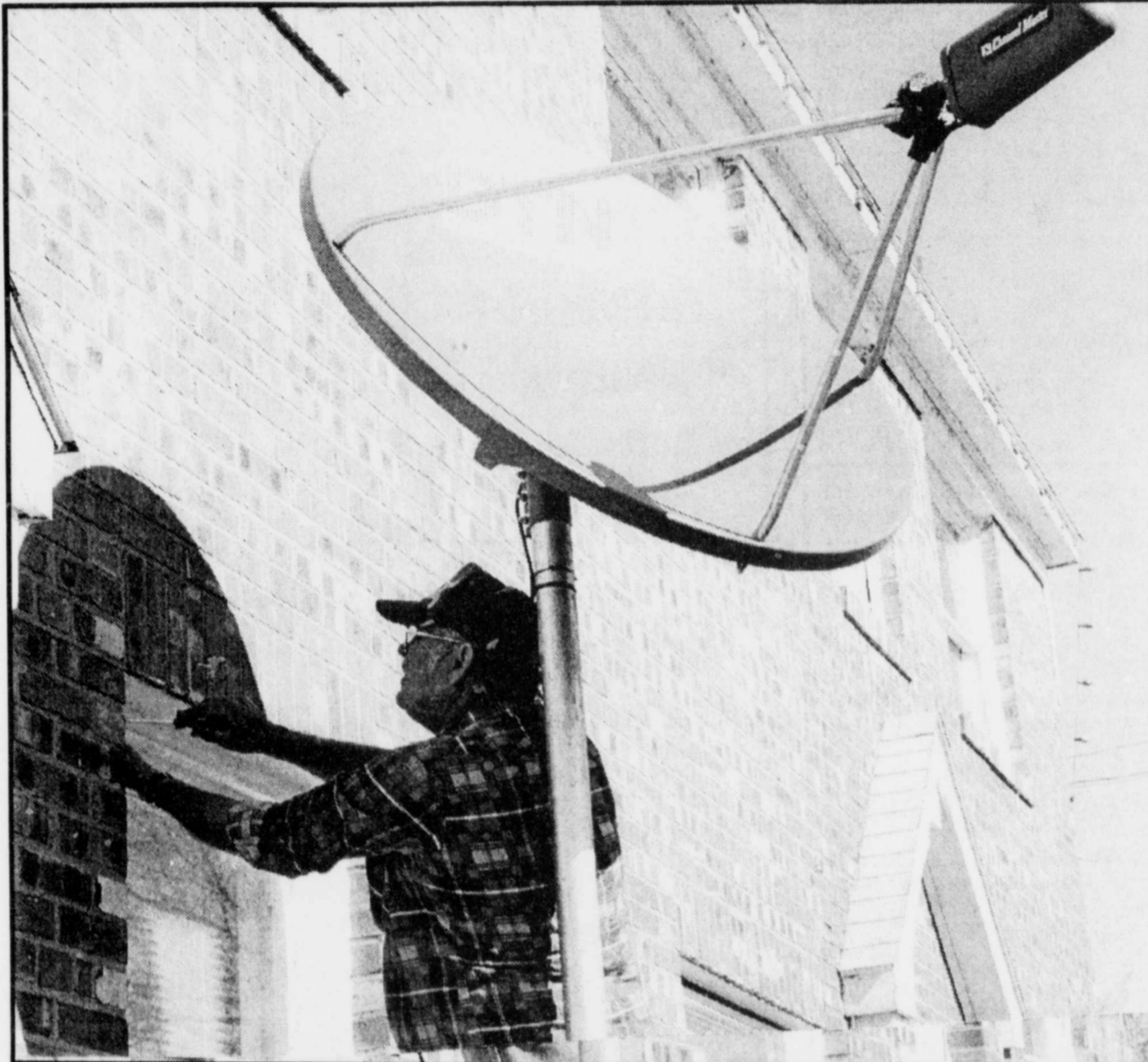
NEW SATELLITE SYSTEM- Charlie Huey worked on the installation of a new satellite system last Tuesday in Talco city hall. The system will provide citizens of Talco with the very latest weather information twenty-four hours a day. According to Fire Chief Randy Carroll the system will be used for storm watchers when threatening weather approaches the city. The system can provide information much faster than depending on other sources can observe threatening weather and relay that information to storm watchers in Talco.
