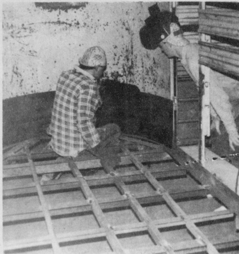
NEW FLOOR—James Hampton and Scott Yancey, both members of the Rivercrest FFA Chapter, install a new metal
