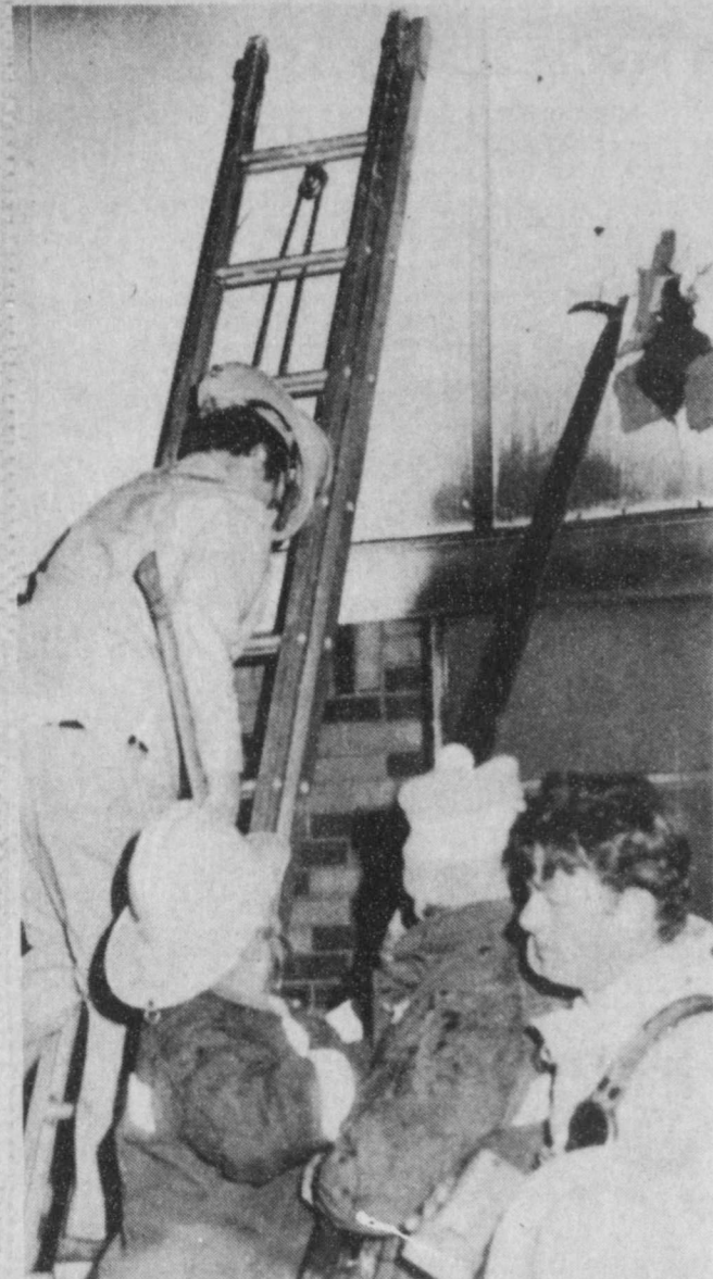
VENTING —Firemen vented the attic on the outside of the building when they arrived at the fire Thursday night. Both Deport and Pattonville volunteers worked to save the building, which suffered little structural damage. (Staff Photo)
