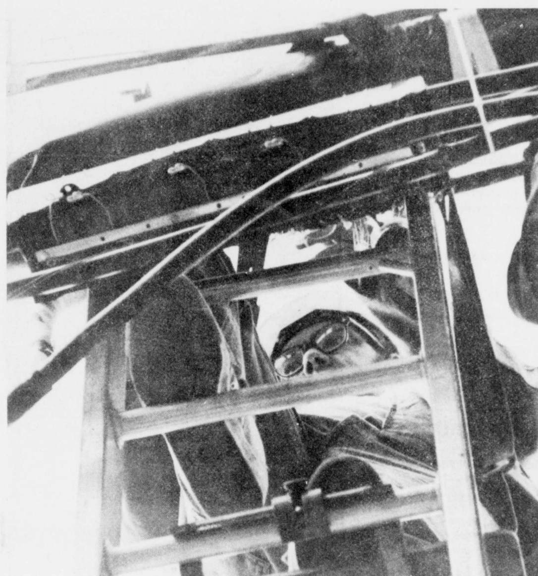
UPGRADING — George Glover, a cable splicer from Garland, makes connections in telephone lines near
