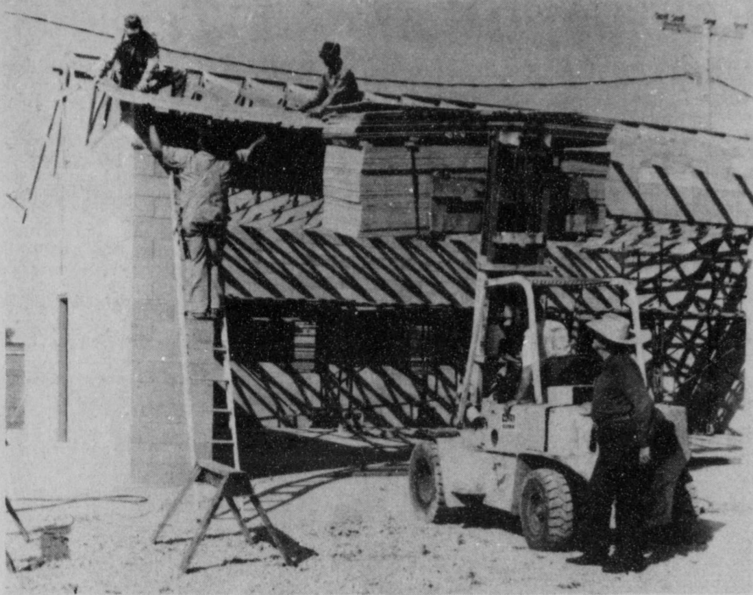
GOING UP —A new three bay garage for repair and maintenance of automobiles is being built at Discount
