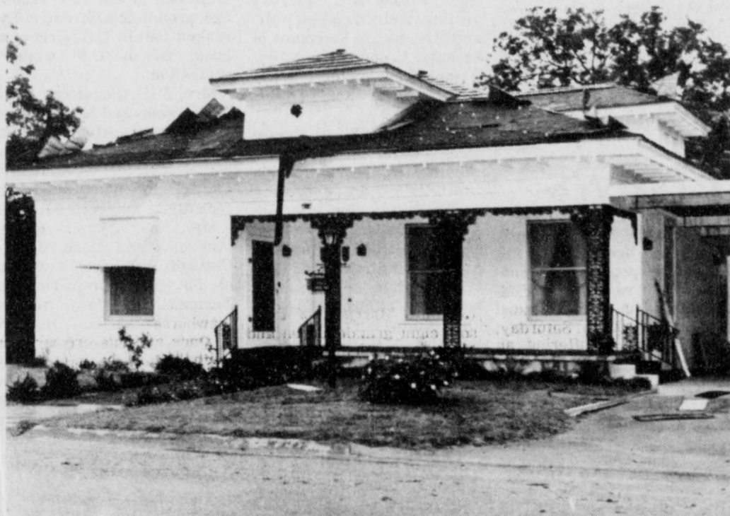
PEELED ROOF —Bogata Funeral Home lost its roof and the upstairs windows blew out when the Saturday night storm hit town. The manager, Jim Wood, was inside the building at the beginning of the storm. A structural crack appeared in the front roof line and the power supply was knocked out. (Staff Photo).
