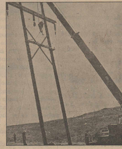
"We're putting in a new 115,000 volt line . . . gives us another feed to back up our dependability . . ."
