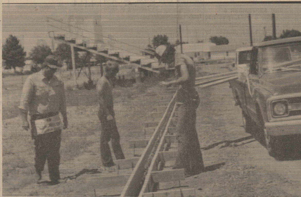
Curbing is being run for the track which is being constructed around the Silvertown School football field. The bleachers have been moved back to make room for the track, the building of which is being done by Fogerson Lumber & Supply, with Stan Fogerson in charge. He is being assisted in the work by Jeff Tiffin and Ken Sarchet.
