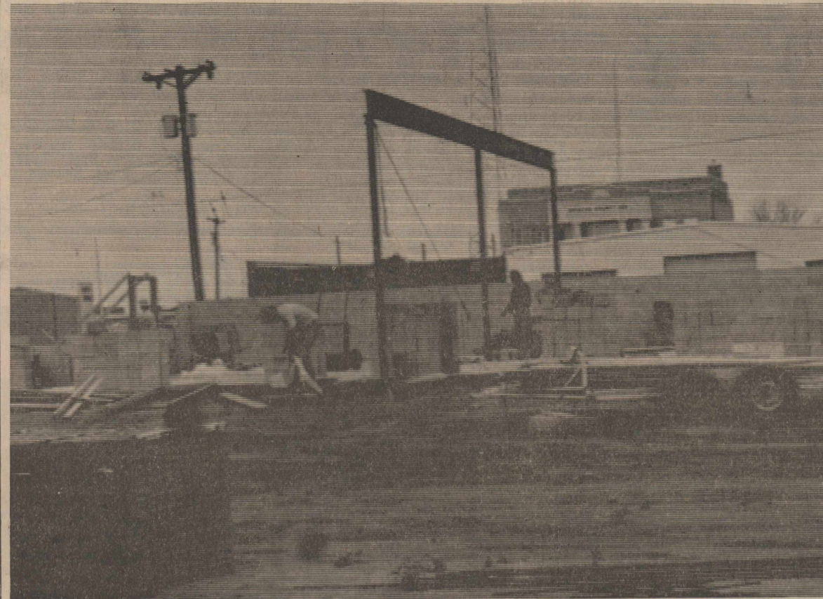
Work is progressing this week on the new Highway 86 just east of Hester and Son Service Center.
