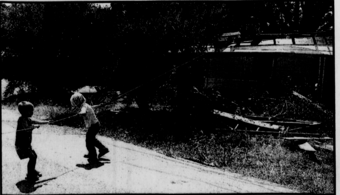
MIGHTY KIDS! Julia Grossman and Johnathan Folsie give a huge heave-ho to pull down the old house over on Depot Street in Deport. The youngsters got a big kick out of helping to tear the derelict structure back. They were carefully supervised and holding on to a long rope to make sure they came to no harm. (Staff Photo by Nanalee Nichols)
