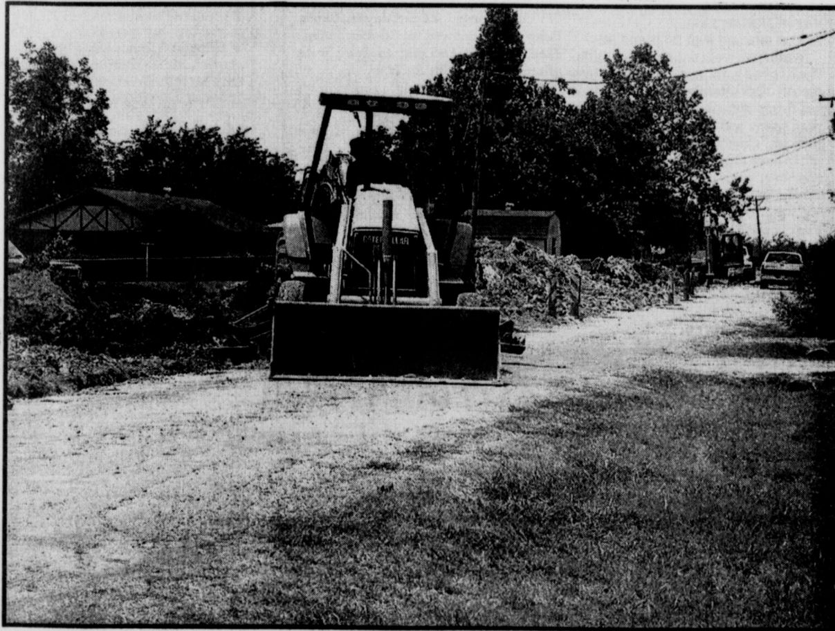
WATER AND SEWER work has been going on in Deport all over town as a grant has provided the funds for new lines which will help provide better water for the town. (Staff Photo by Nanalee Nichols)
