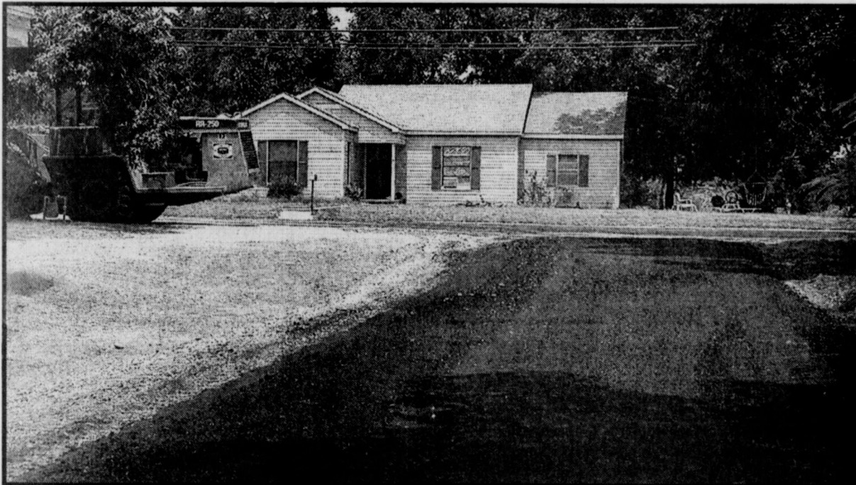
ROAD WORK-Lamar County Pct. 1 has been paving a number of streets in Deport, under contract with the City of Deport to do so. Fourth Street and second street are among streets that had been gravel that now have an oil topping. (Staff photo by Nanalee Nichols)
