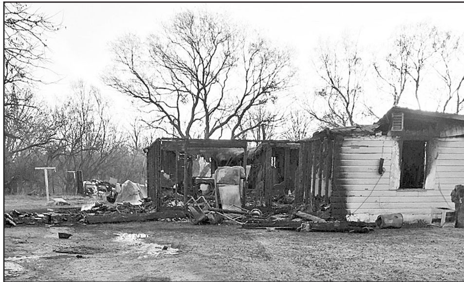
HOUSE FIRE —The Haskell Volunteer Fire Department responded to the call of a house fire at 1408 N. Ave. B Tuesday night, Dec. 13.
