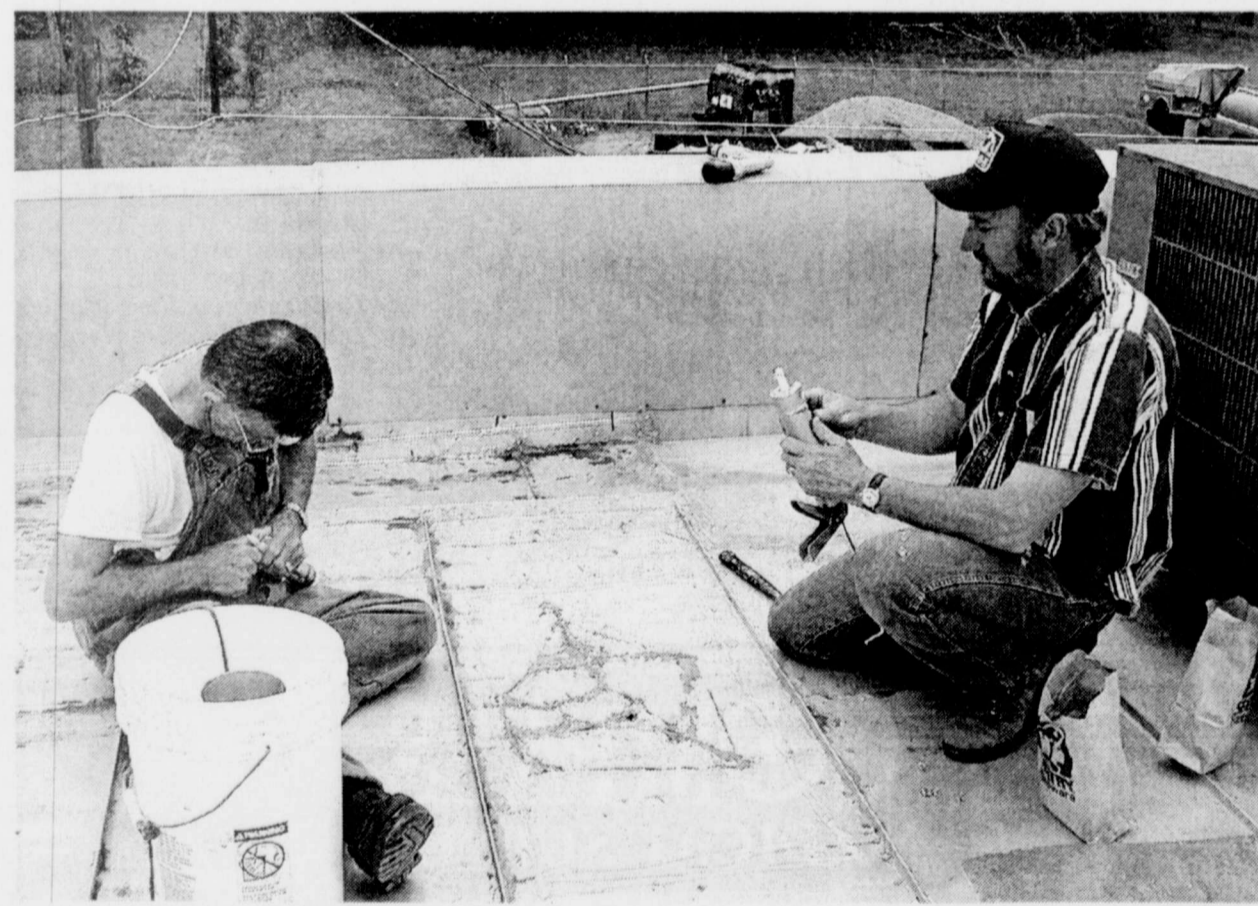
PATCH JOB-Duane Glover and son-in-law Jerome Chapman patch the roof of City Drug Store Sunday afternoon after someone crawled up on the roof and cut a hole in the drug store roof and the Deport Times roof. The would be thieves did not gain access to the buildings, but a heavy rain afterward resulted in lots of water pouring into them. Lamar County Sheriffs deputies have the matter under investigation.
