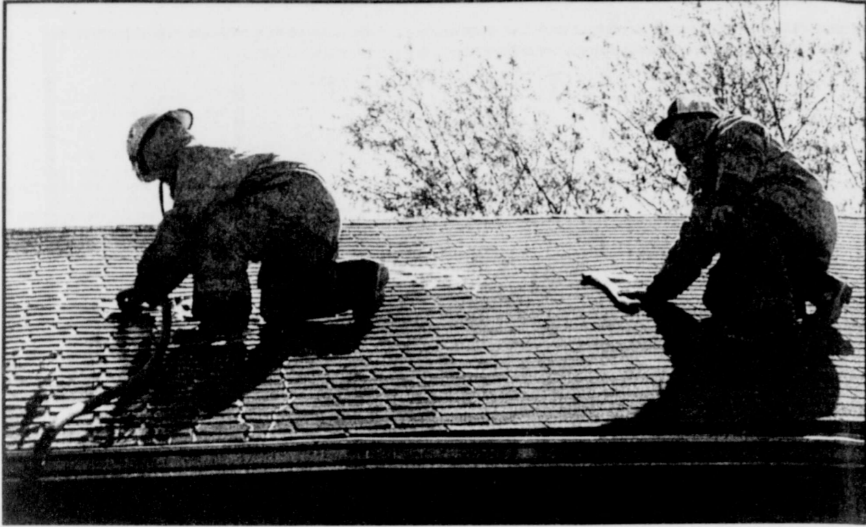
ON THE ROOF -Mike Francis and Thomas Nichols of the Deport Volunteer Fire Department pour water into the attic of Larry and Judy Whittle's home last Thursday. A close look will show the portions of the room where the heat had curled the shingles. The Whittle home suffered severe damage in the blaze. Fire departments from Cunningham, Deport, Pattonville and Blossom brought the blaze under control. (Staff Photo by Nanalee Nichols)
