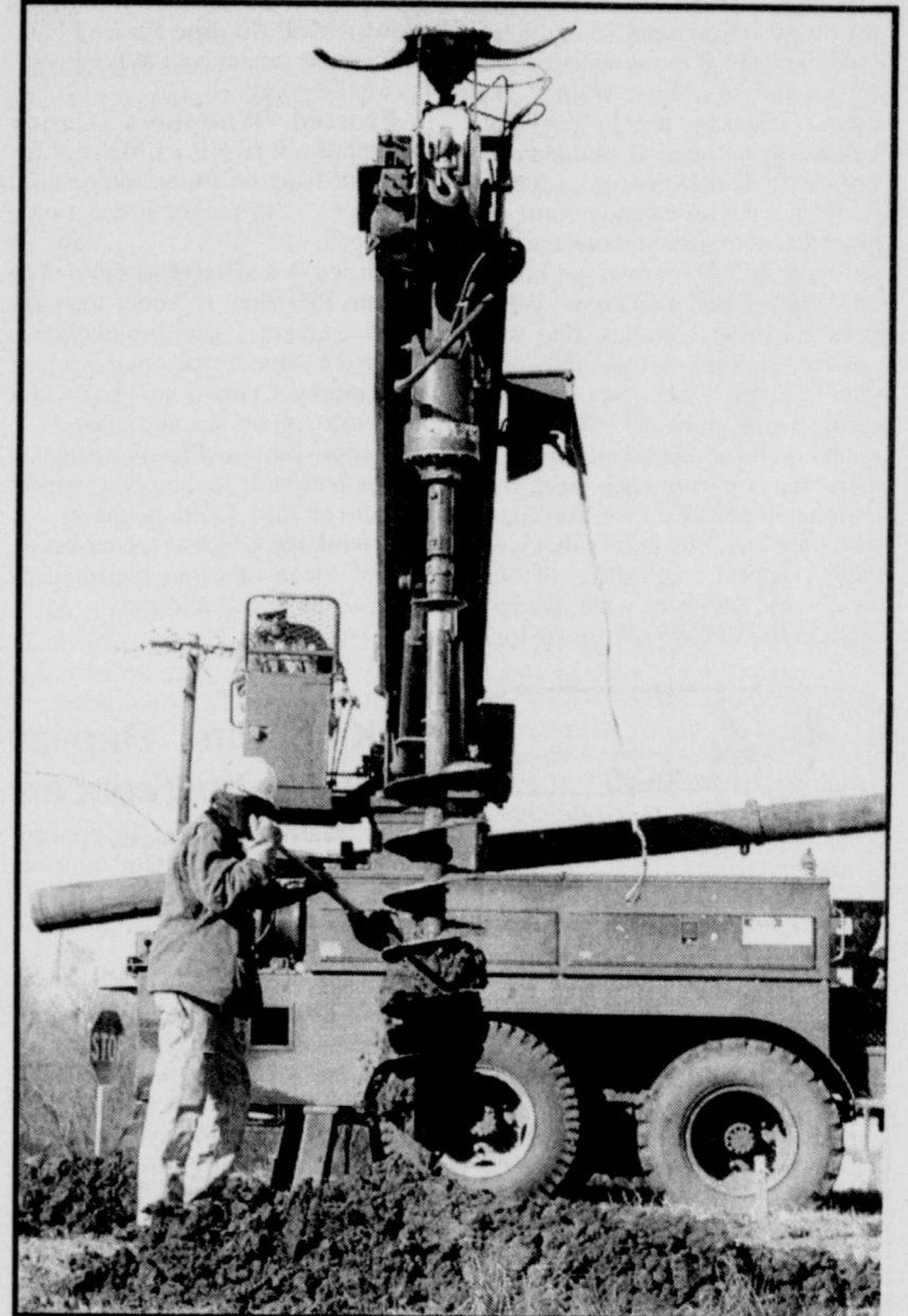
THANKS AGAIN - Kenneth Palmer & Tommy Childress of Texas New Mexico Power Company drill holes one more time for the Main Street Sign at the intersection of Main St. & Highway 271.
